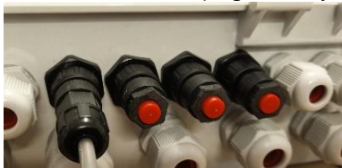
Figure 65 – Only one device connected, 3 plugs.
